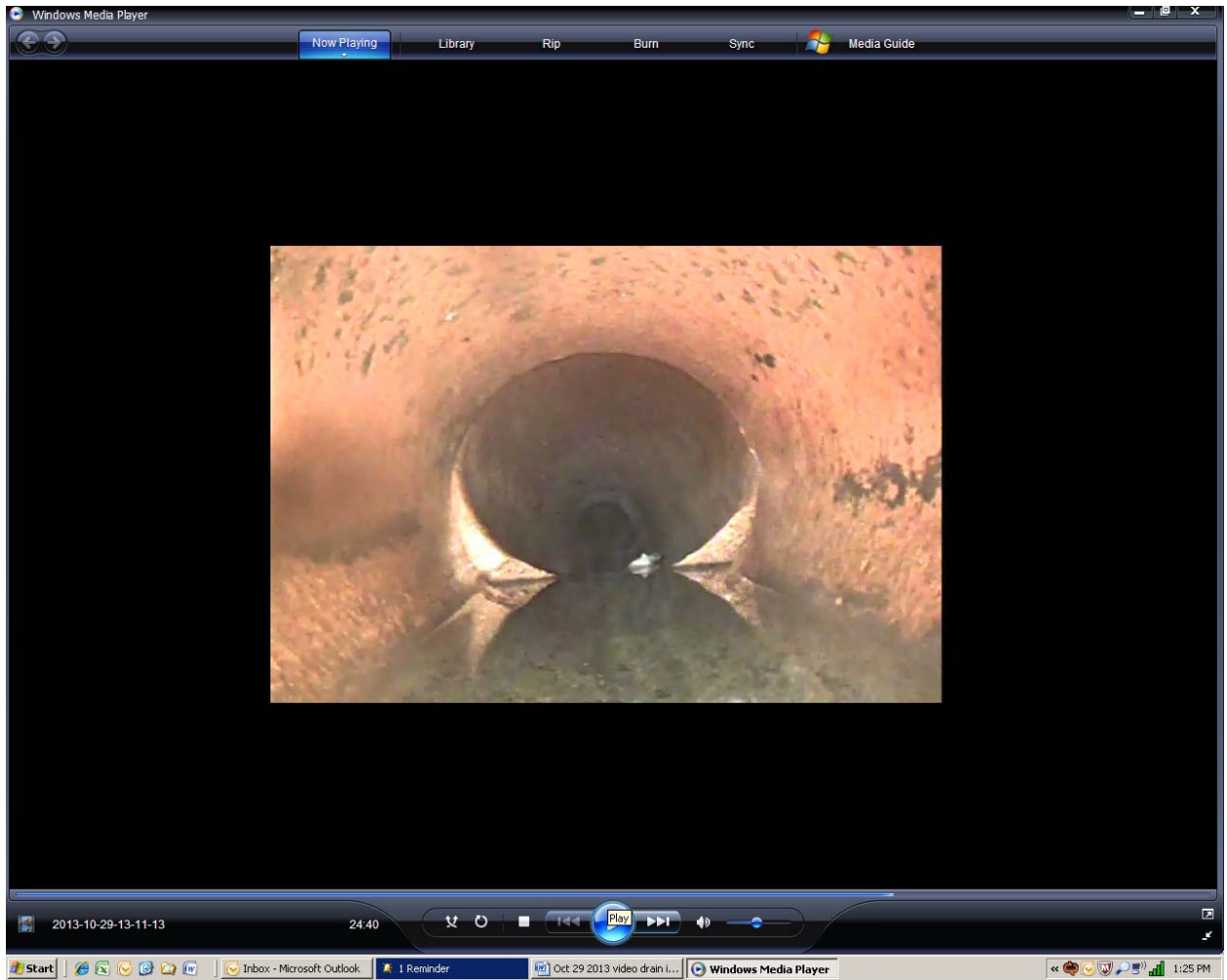
Screen shot 16: separated joint in four-inch clay pipe drain line 6 at approximately 34 feet
