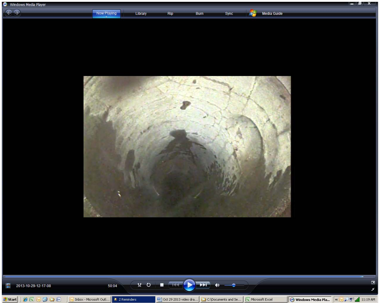
Screen shot 3: connection from drain line 1 (right side) at 11 feet in eight-inch clay pipe drain line 2, note cracks in top of pipe
