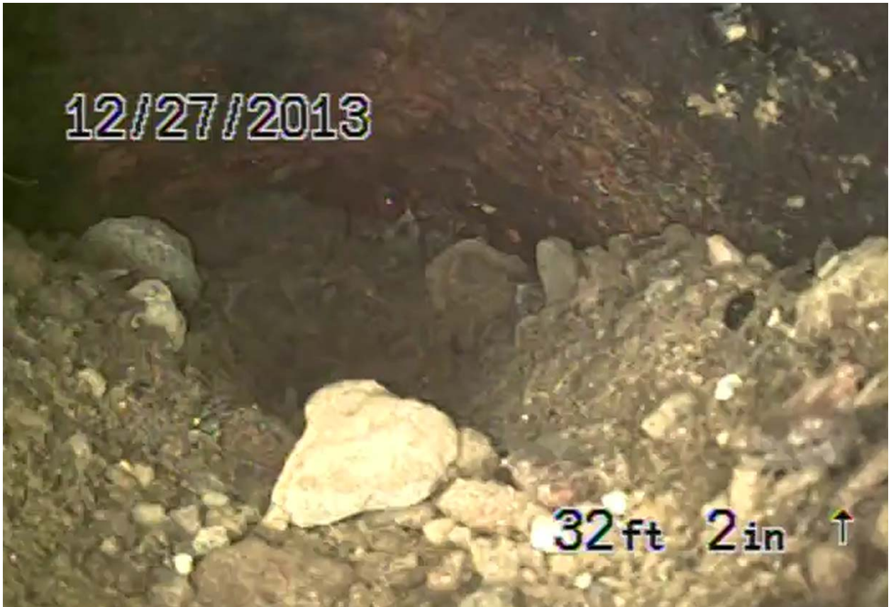
Screen shot 23: four-inch cast iron pipe drain line 7 filled with soil at the extent of inspection approximately 32 feet from the former inspection sump
