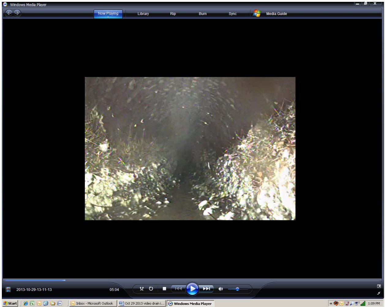
Screen shot 19: four-inch clay pipe drain line 6 with significant root penetration in pipe
