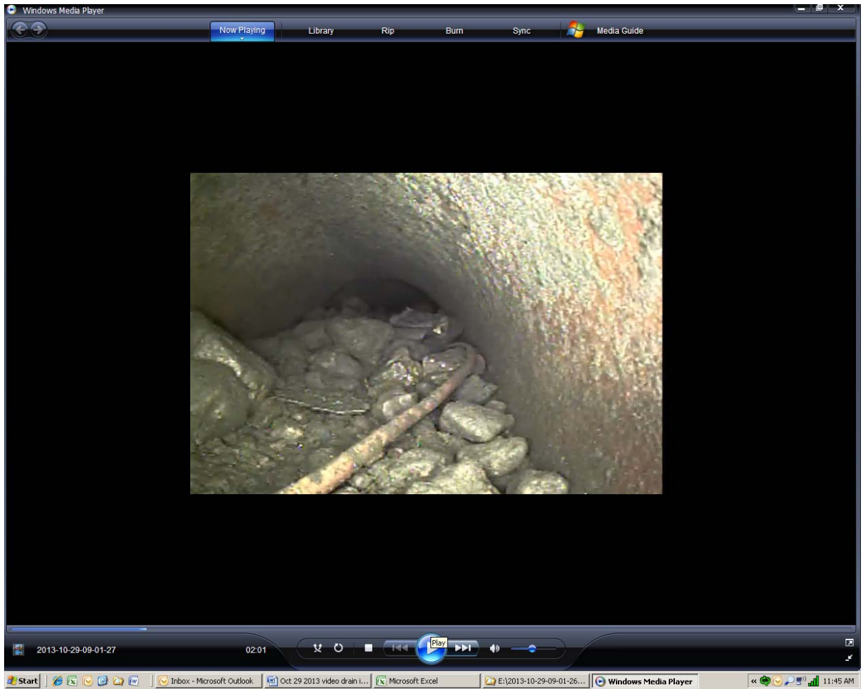
Screen shot 7: section of four-inch clay pipe drain line 4 with sediment and gravel
