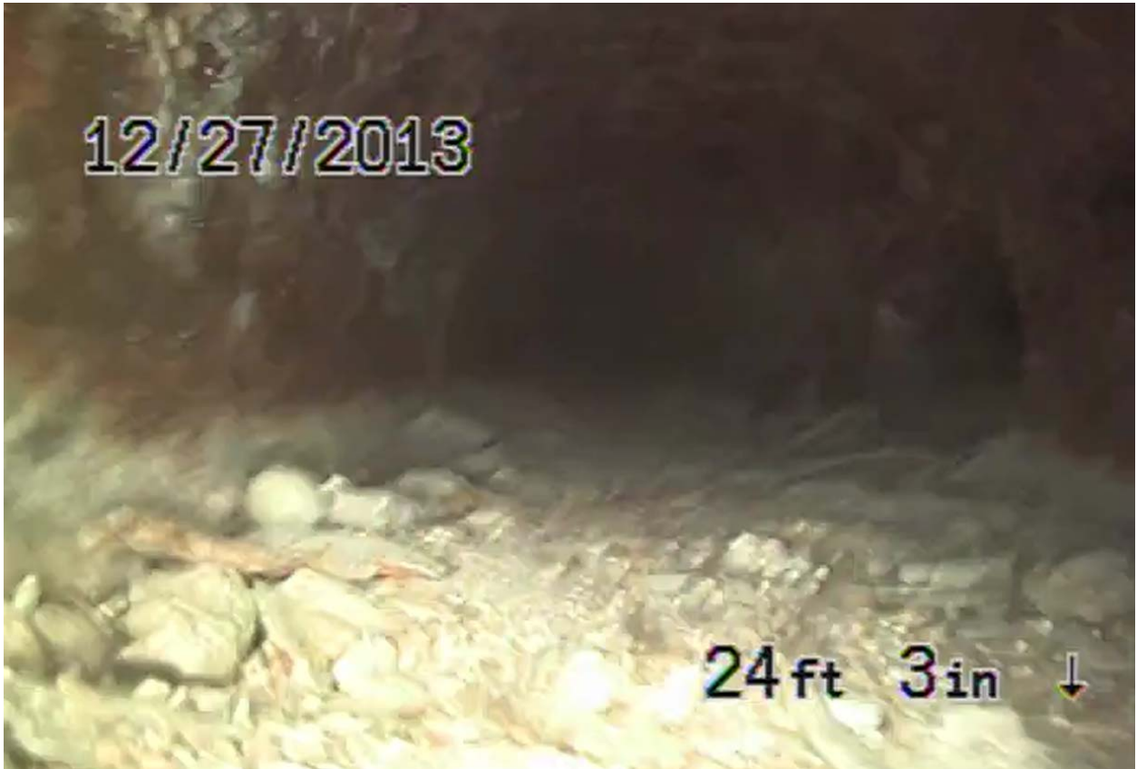
Screen shot 27: four-inch cast iron pipe drain line 8 beneath Building 3 with potential connection on the right
