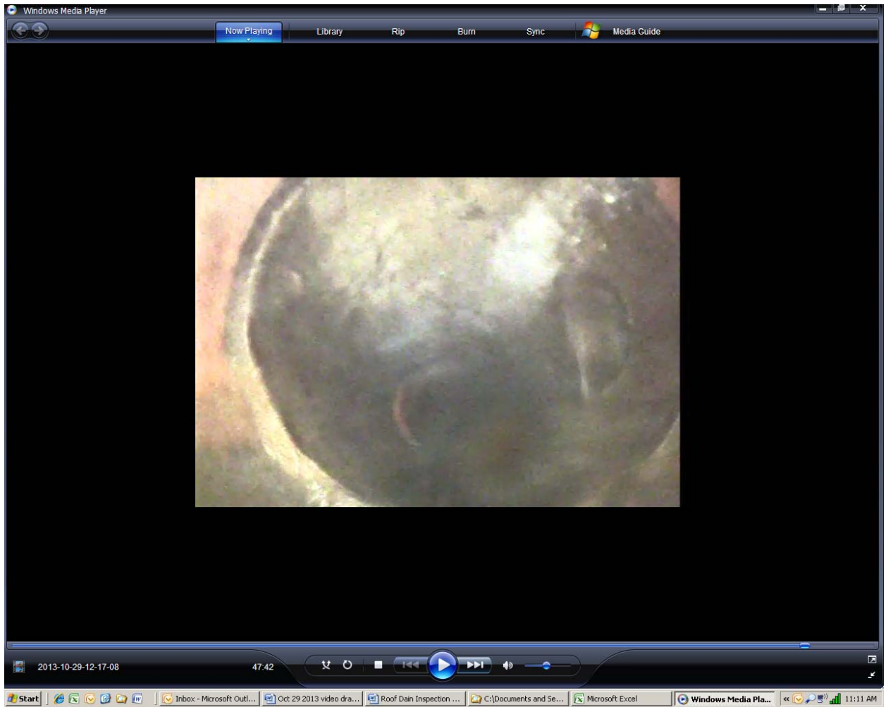
Screen shot 4: unknown connection (right) at approximately 50 feet in eight-inch clay pipe drain line 2
