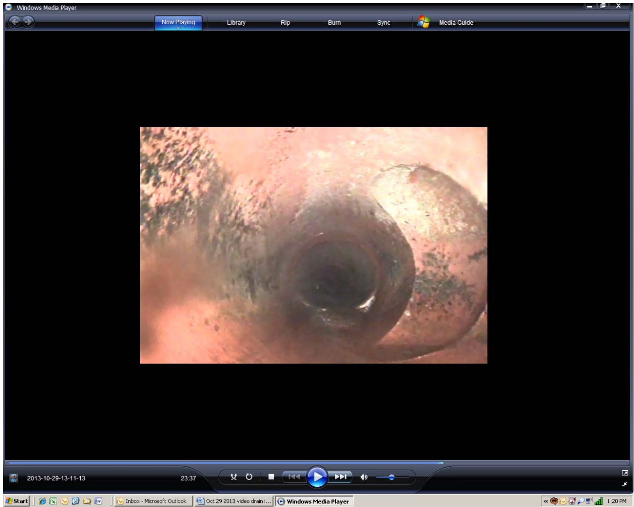
Screen shot 15: connection to four-inch clay pipe drain line 6 at approximately 28 feet (subsequently confirmed to be former Building 3 waste water line), also note off-set joint just past connection
