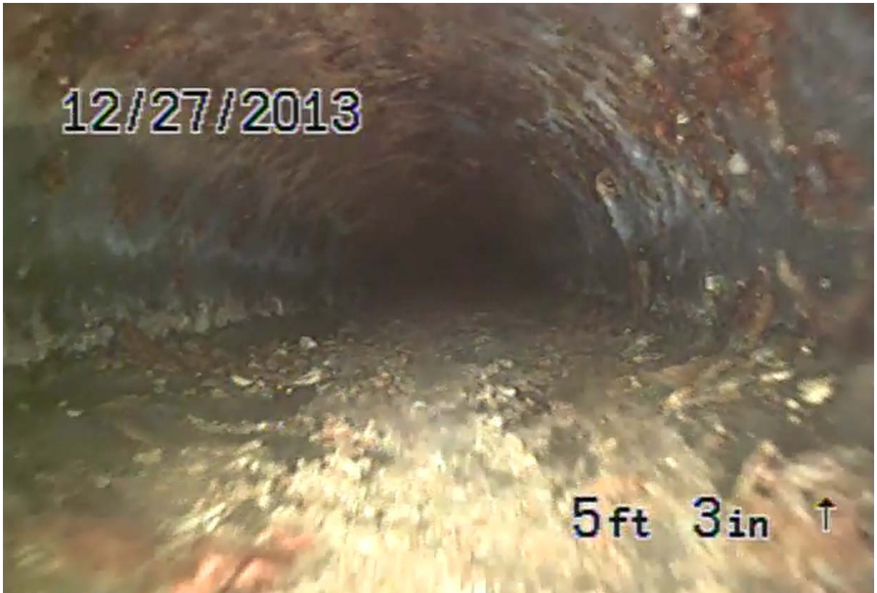
Screen shot 25: four-inch cast iron pipe drain line 8 heading south beneath Building 3
