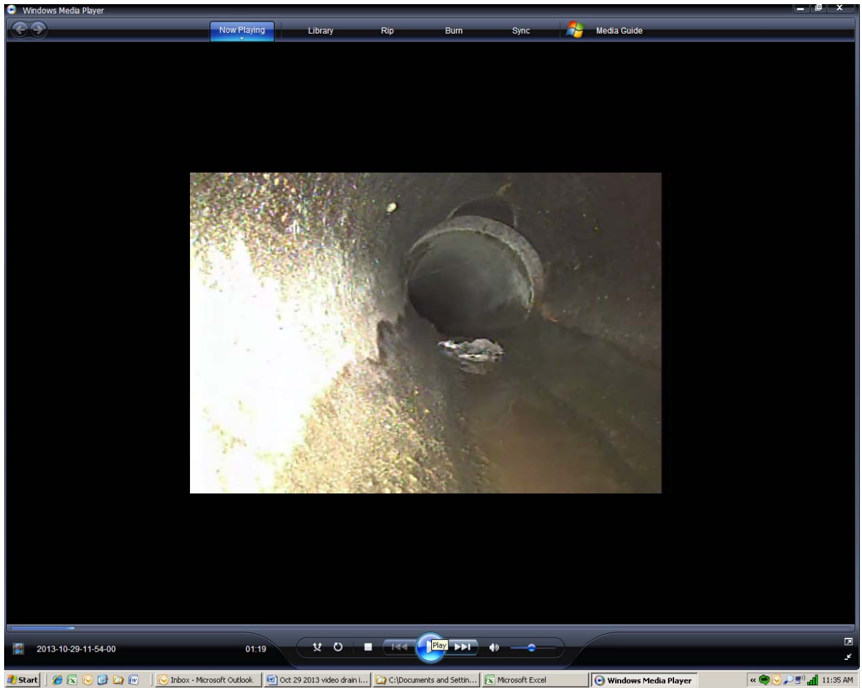
Screen shot 5: off-set pipe joint in four-inch clay pipe drain line 3
