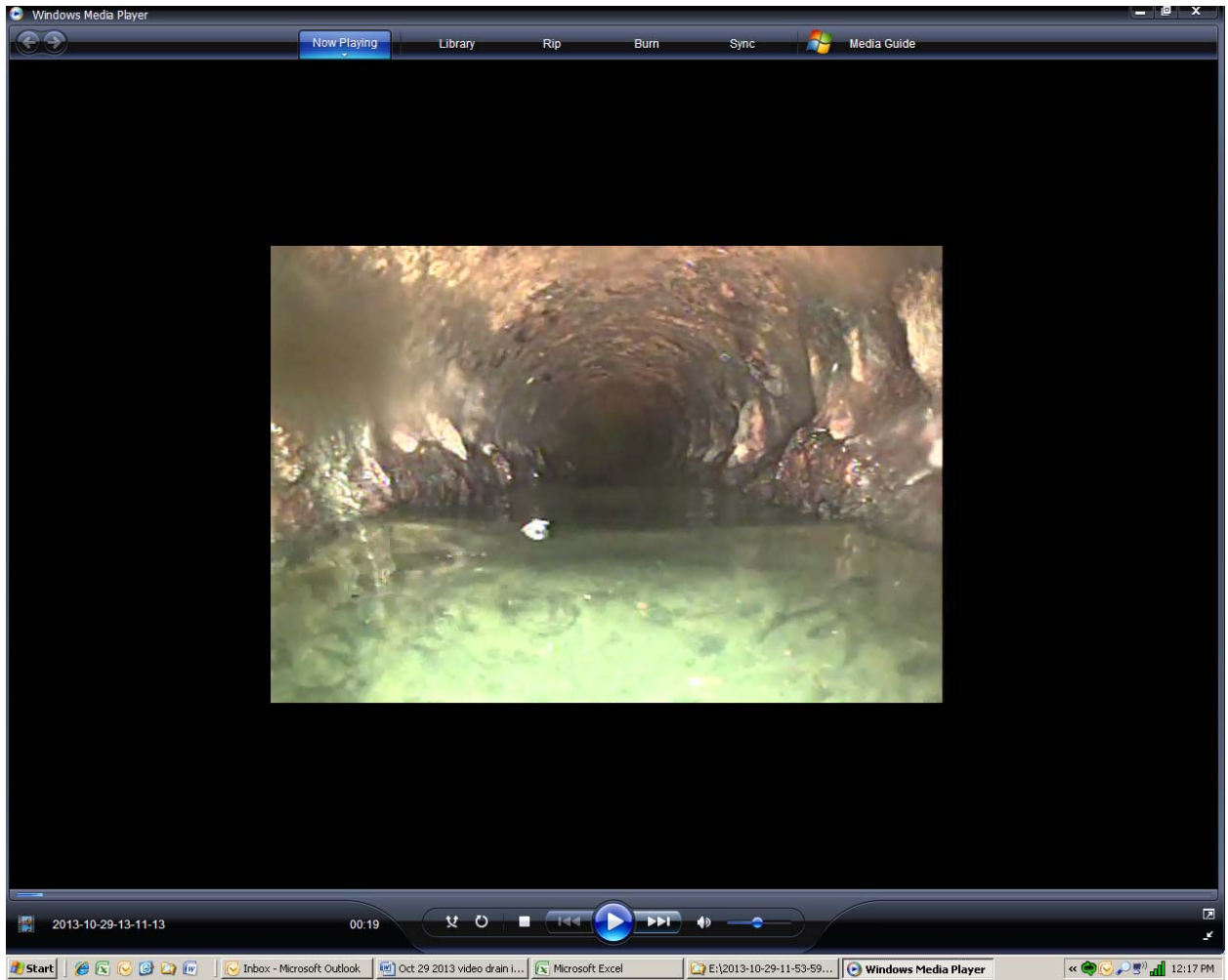
Screen shot 13: Initial section of four-inch cast iron pipe drain line 6 outside of building with water and significant corrosion
