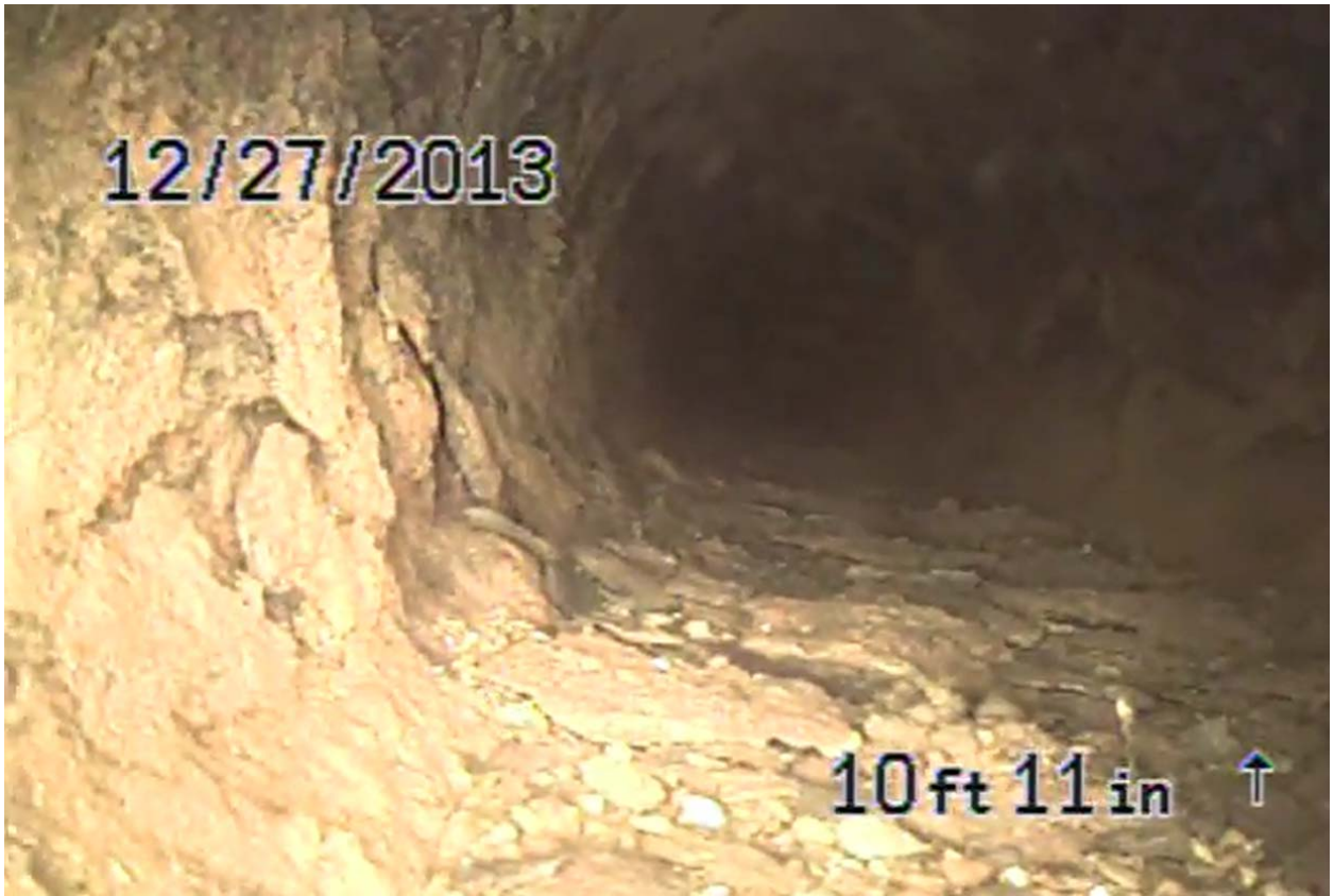
Screen shot 20: four-inch cast iron pipe drain line 7 with wall deposits and sediment
