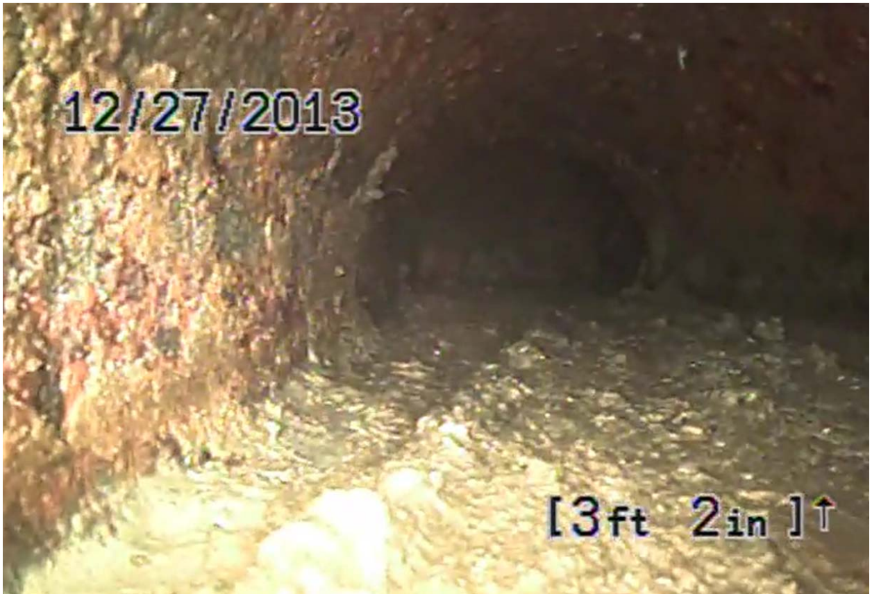
Screen shot 24: four-inch cast iron pipe drain line 8 heading north to Drain Line 6
