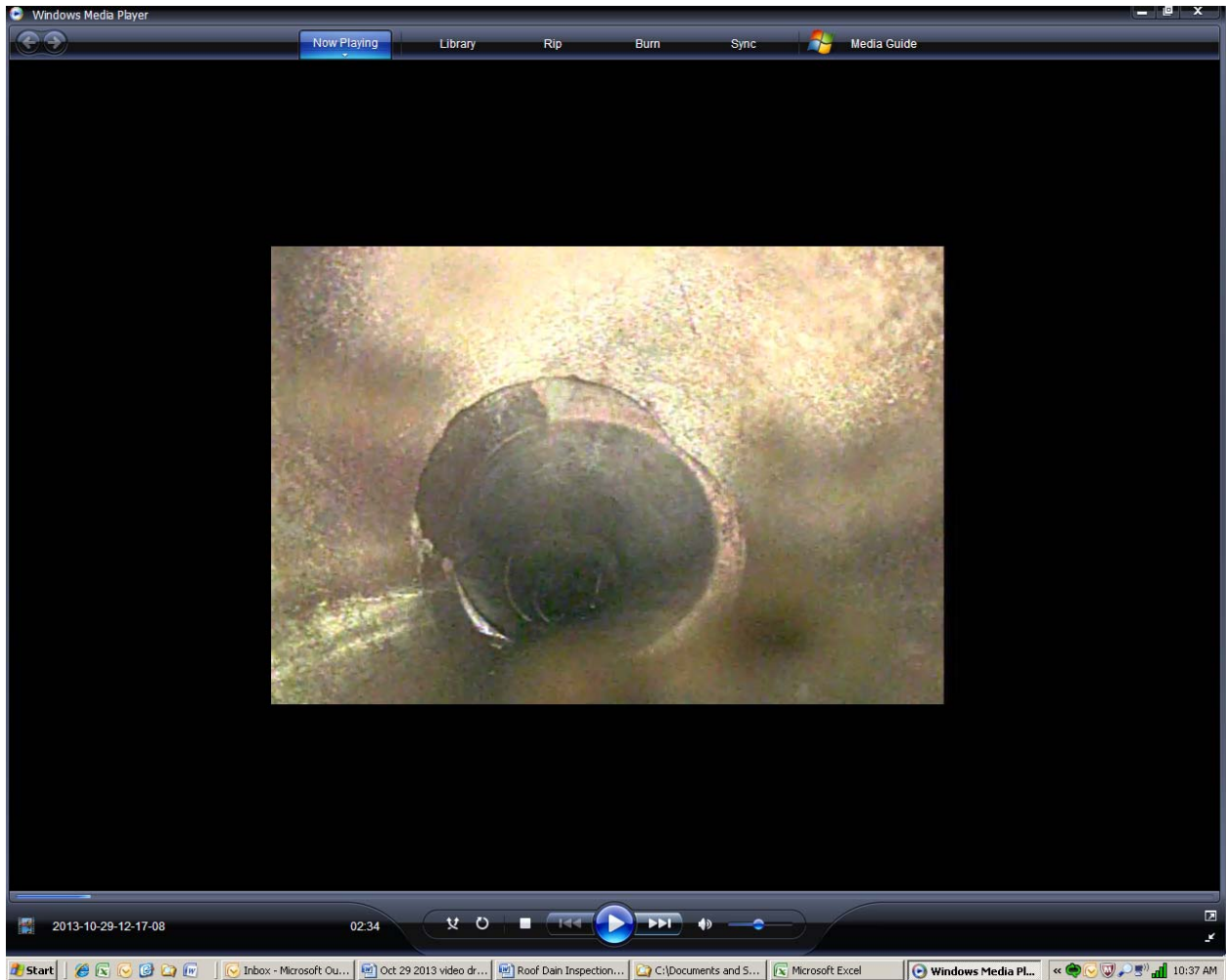
Screen shot 1: broken bell connection (upper left) at 91 feet in eight-inch clay pipe drain line 2
