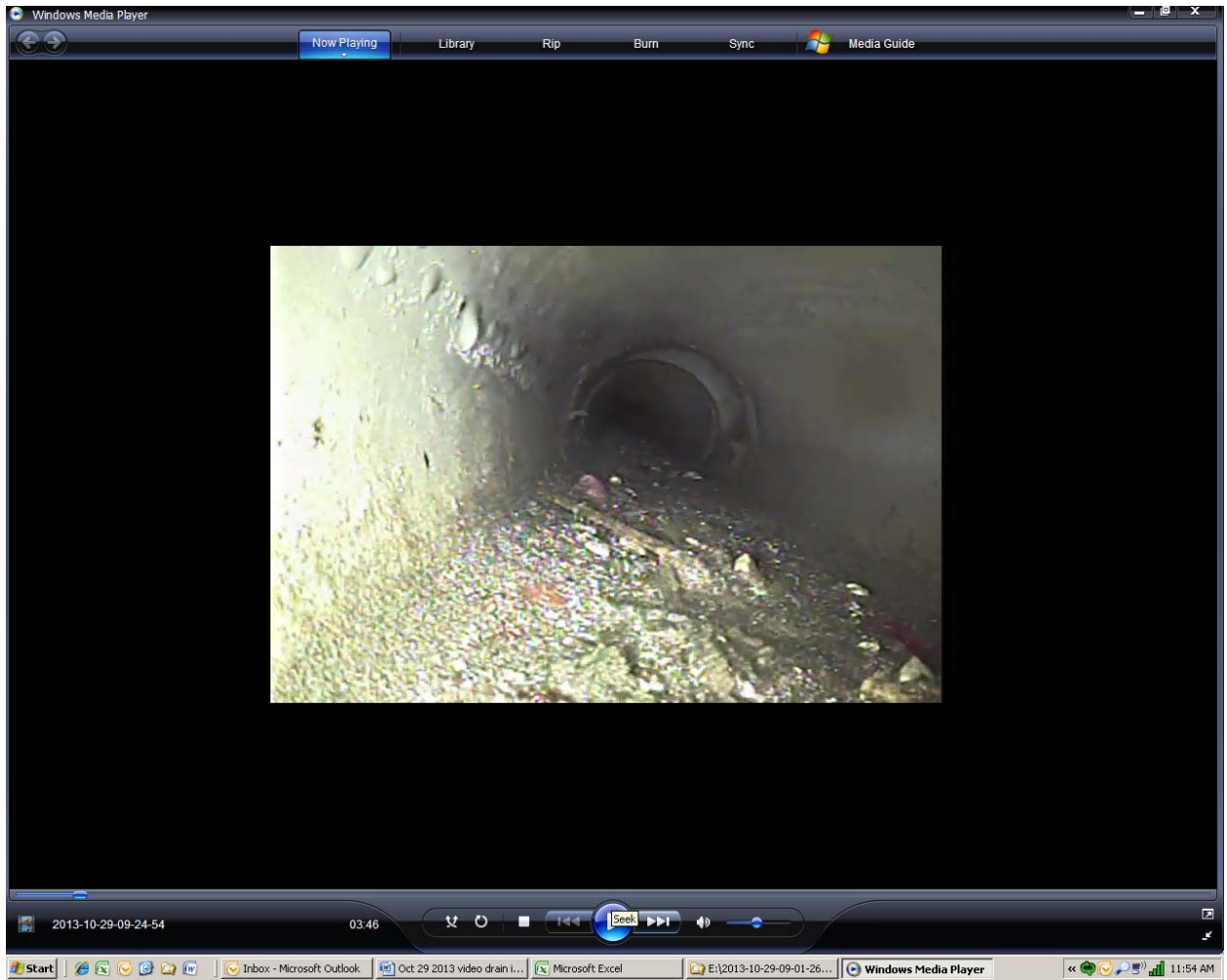
Screen shot 9: sediment in initial section of four-inch PVC pipe drain line 5, note blistering of PVC on the upper left
