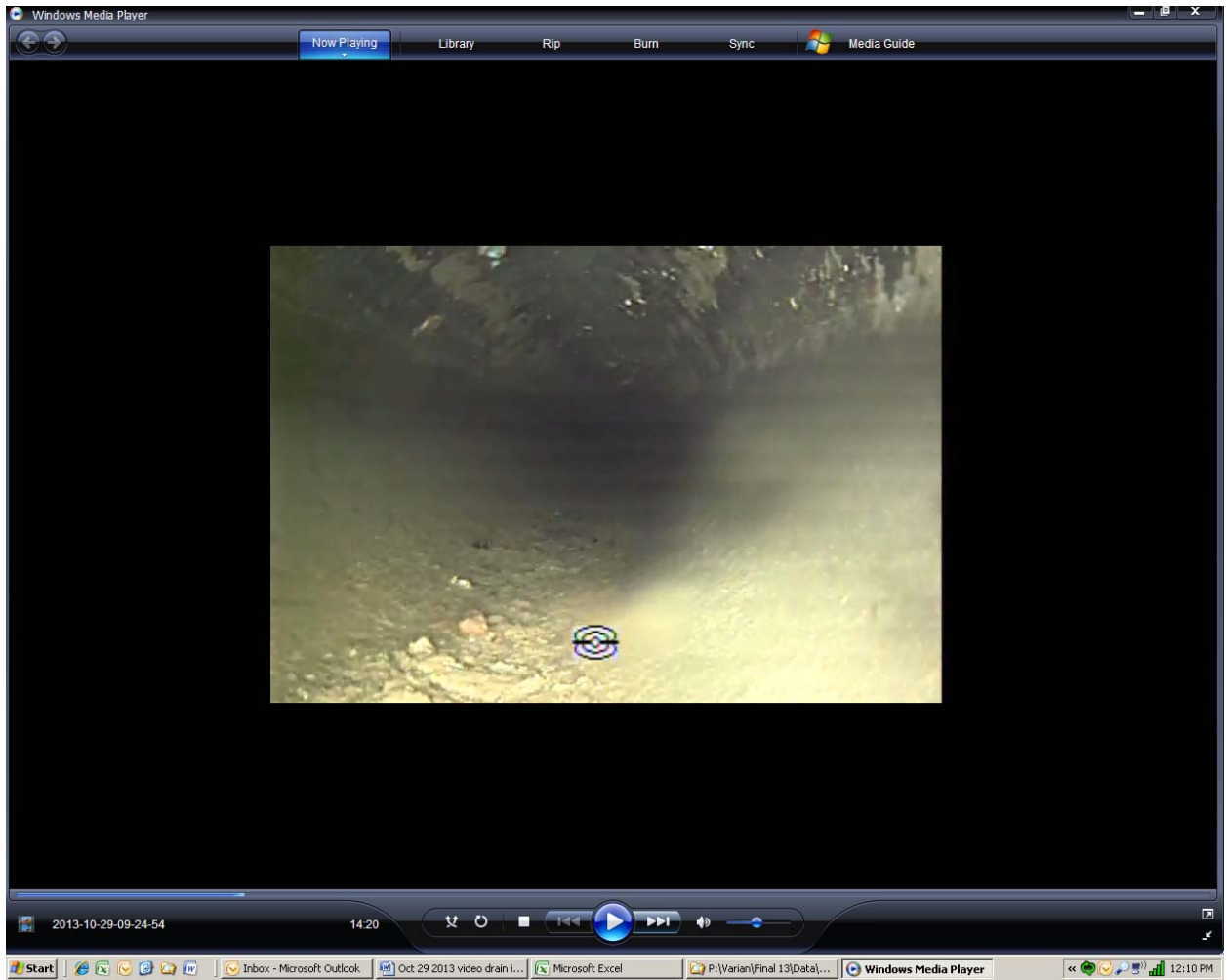
Screen shot 12: section of four-inch PVC pipe drain line 5 outside of building filled with water
