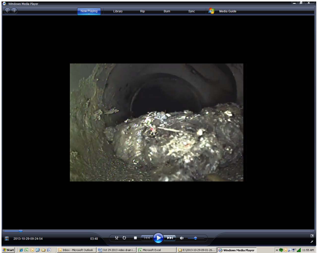
Screen shot 10: debris and potential connection (upper right) to four-inch PVC pipe drain line 5 at approximately four feet
