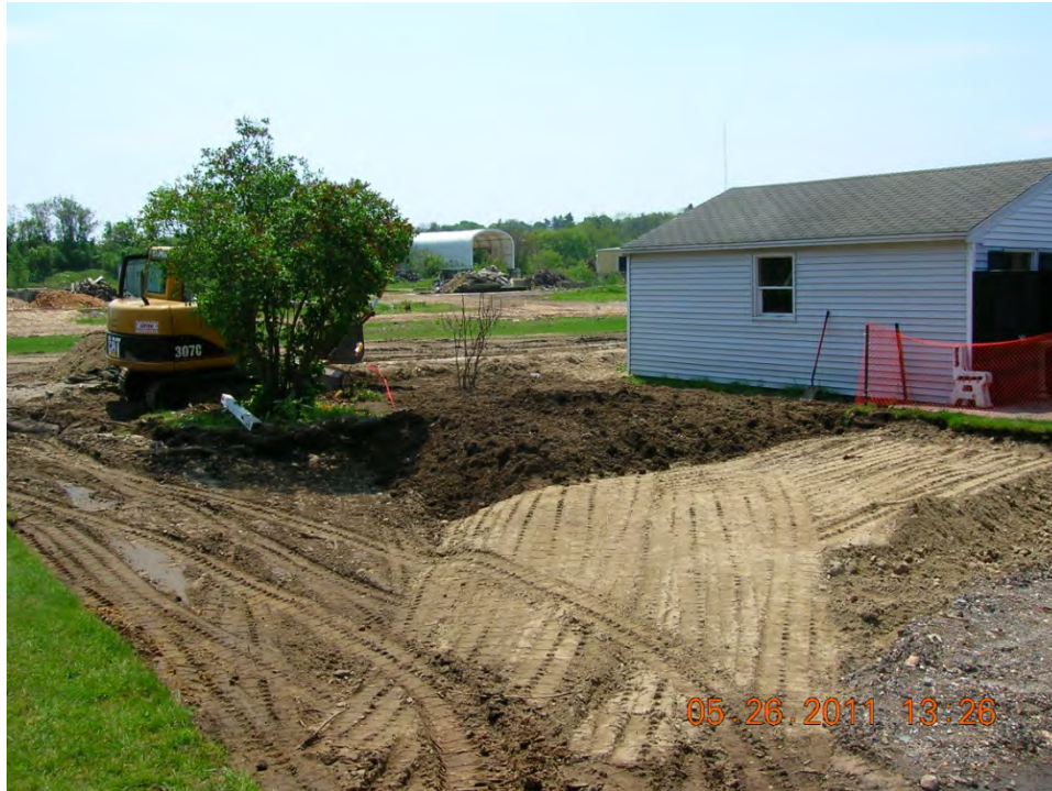
SCENE: View of site restoration activities in the side yard at 41 Hoffman Avenue. Photograph taken facing south.
