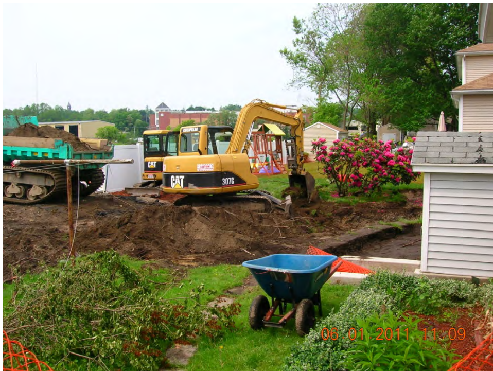
SCENE: View of excavation activities in the backyard at 41 Hoffman Avenue. Photograph taken facing west.
