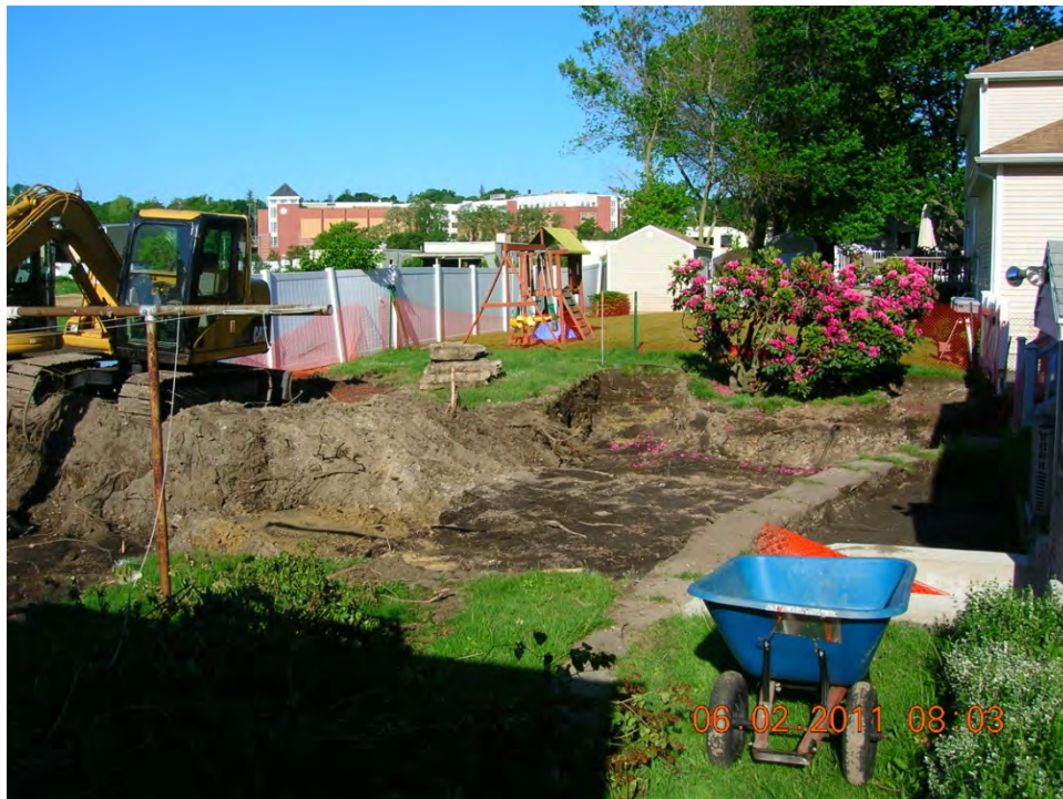
SCENE: View of excavation activities in the backyard at 41 Hoffman Avenue. Photograph taken facing west.
