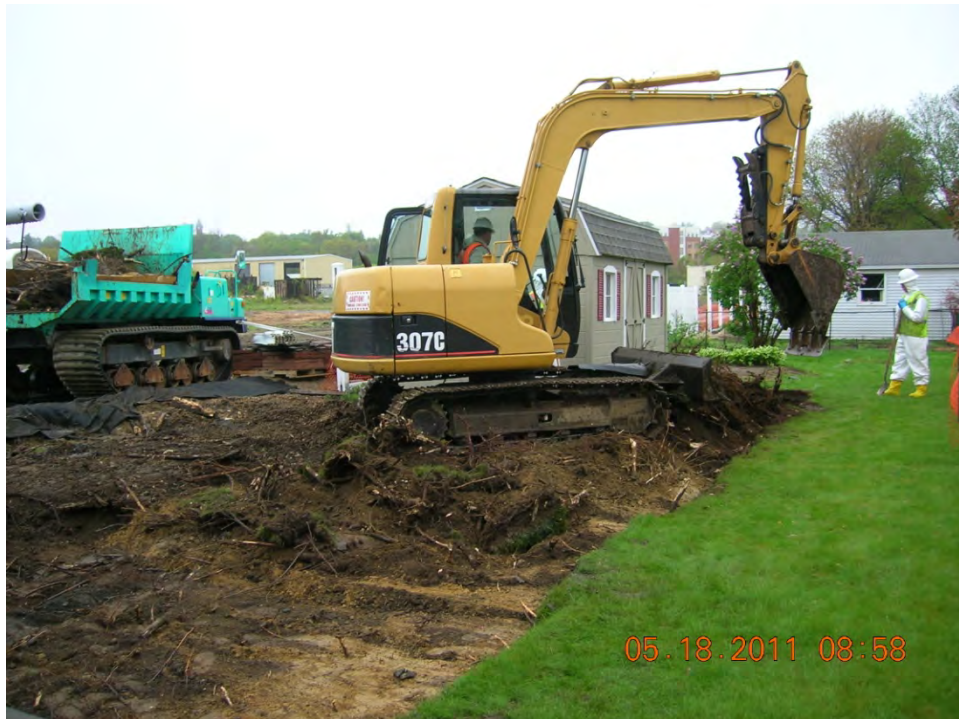
SCENE: View of excavation activities in the backyard at 51 Hoffman Avenue. Photograph taken facing west.
