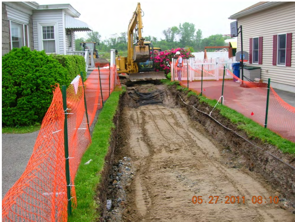
SCENE: View of backfilling activities at 33 Hoffman Avenue. Photograph taken facing south.
