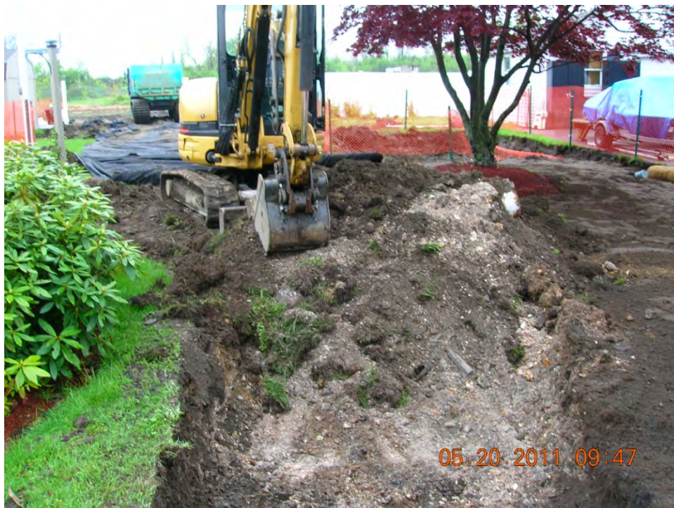
SCENE: View of excavation activities in the side yard at 41 Hoffman Avenue. Photograph taken facing south.
