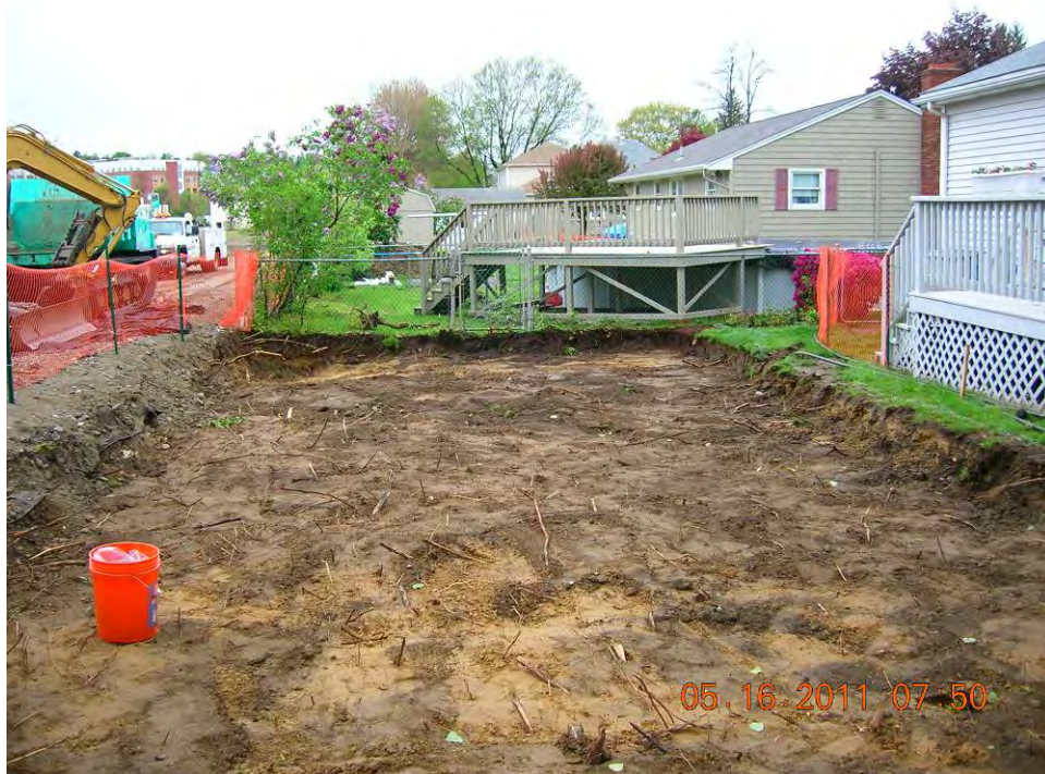
SCENE: View of the excavation in the backyard at 53 Hoffman Avenue. Photograph taken facing west.
