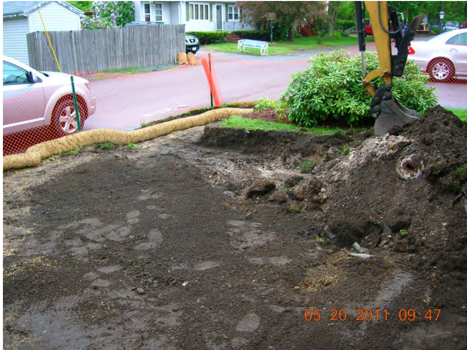
SCENE: View of excavation activities in the side yard at 41 Hoffman Avenue. Photograph taken facing east.
