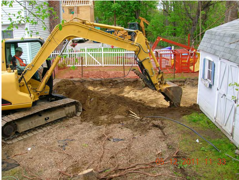
SCENE: View of excavation activities in the backyard at 53 Hoffman Avenue. Photograph taken facing north.
