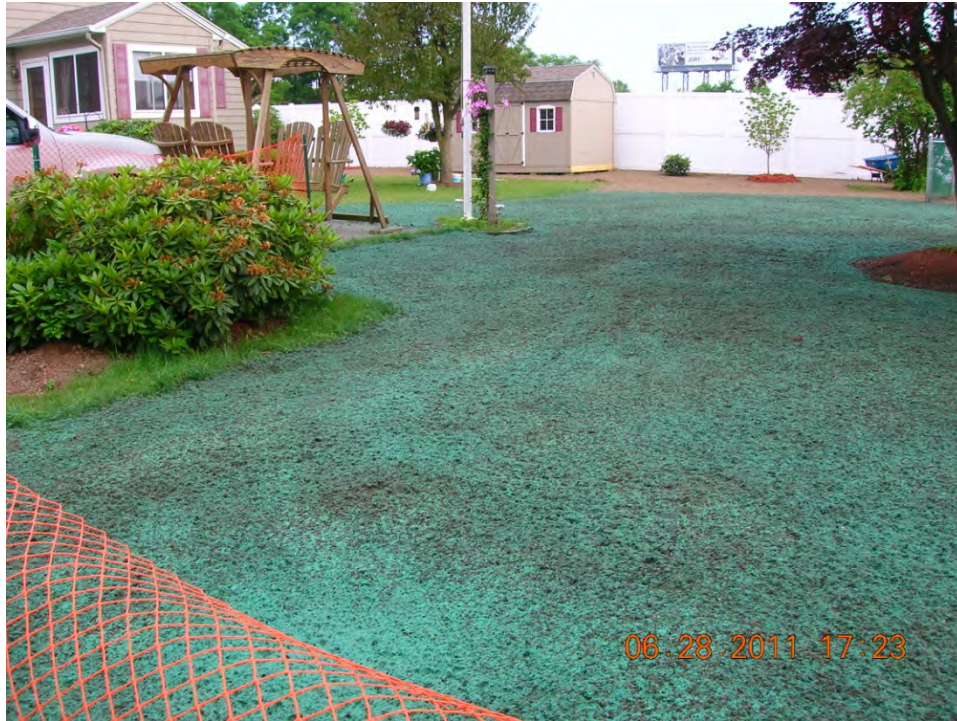
SCENE: View of the restored side yard at 41 Hoffman Avenue. Photograph taken facing south.
