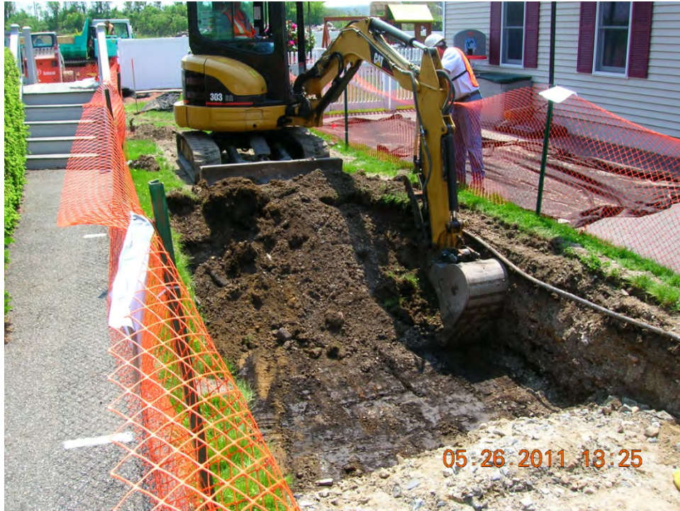
SCENE: View of excavation activities at 33 Hoffman Avenue. Photograph taken facing south.
