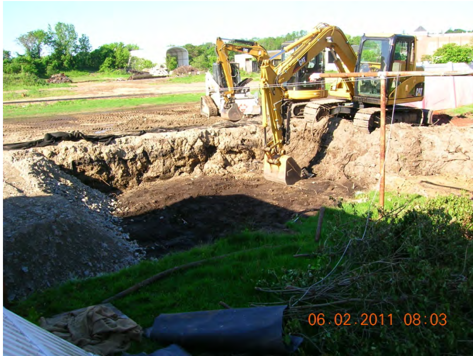
SCENE: View of excavation activities in the backyard at 41 Hoffman Avenue. Photograph taken facing west.
