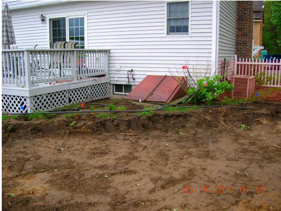
SCENE: View of the excavation in the backyard at 53 Hoffman Avenue. Photograph taken facing north.
