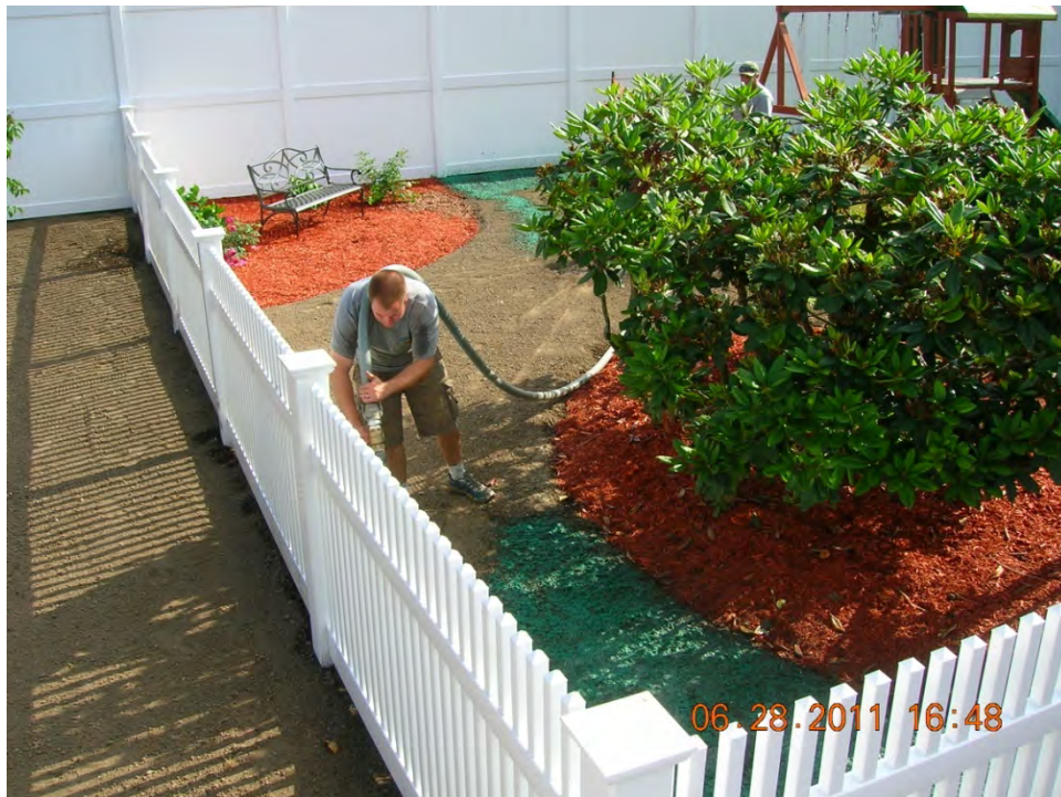
SCENE: View of site restoration activities in the backyard at 33 Hoffman Avenue. Photograph taken facing south.
