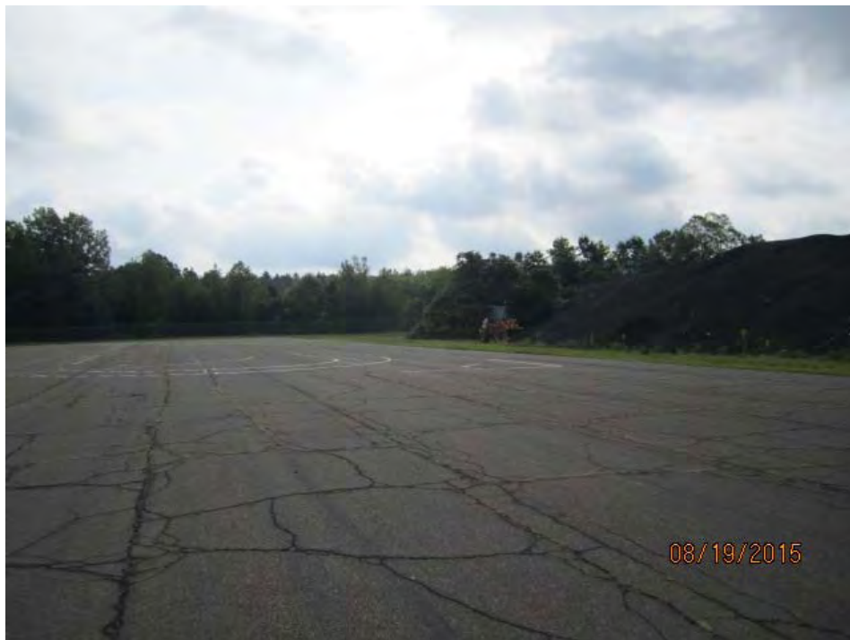
Photo 6: Fire Department Equipment Test Area – East End of Sierra Taxiway
