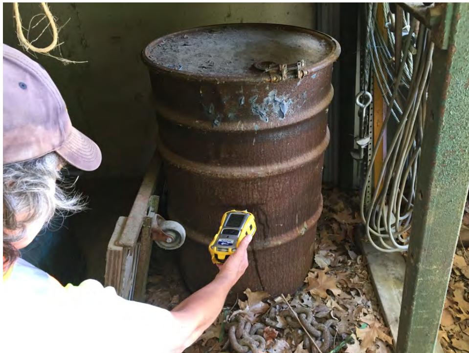
SCENE: View of the rusty, partially corroded 55-gallon steel drum inside the large steel garage/warehouse building. Photograph taken facing northeast. DATE: 23 June 2016 TIME: 1014 hours PHOTOGRAPHER: J. Kelly CAMERA: iPhone 6
