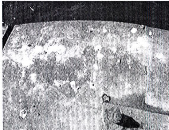
Figure 21 Photo 42 (see Appendix D page 33) showing the cracked top stone confined by the most likely ASR expanding protruding concrete.
