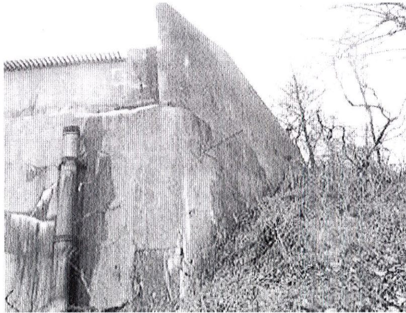
Figure 3 Photo 12 North wingwall at west Abutment with Cracking and Hollow Areas
