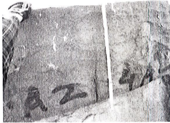
Figure 22 Photo 43 (see Appendix D page 34) showing the cracked top stone most likely from expansion of the protruding concrete.
