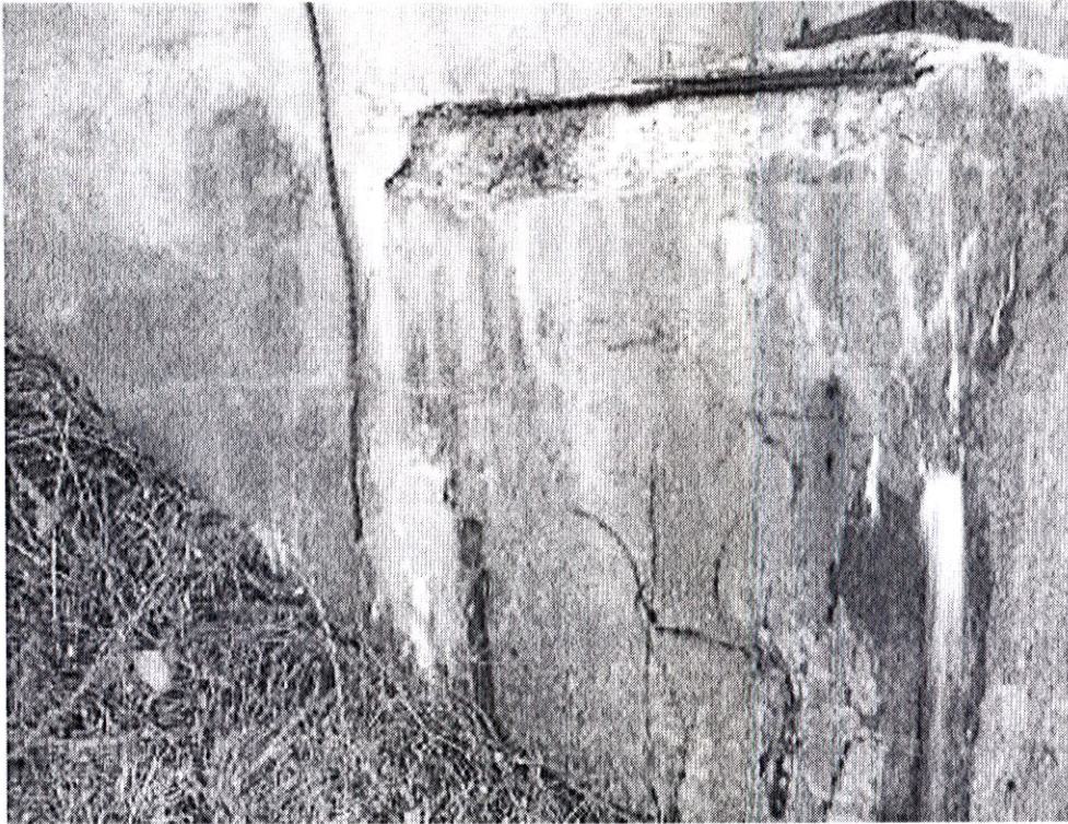
Figure 1 Photo 7 from Appendix D Spall on South End of west Abutment Bridge Seat, Looking Northwest
