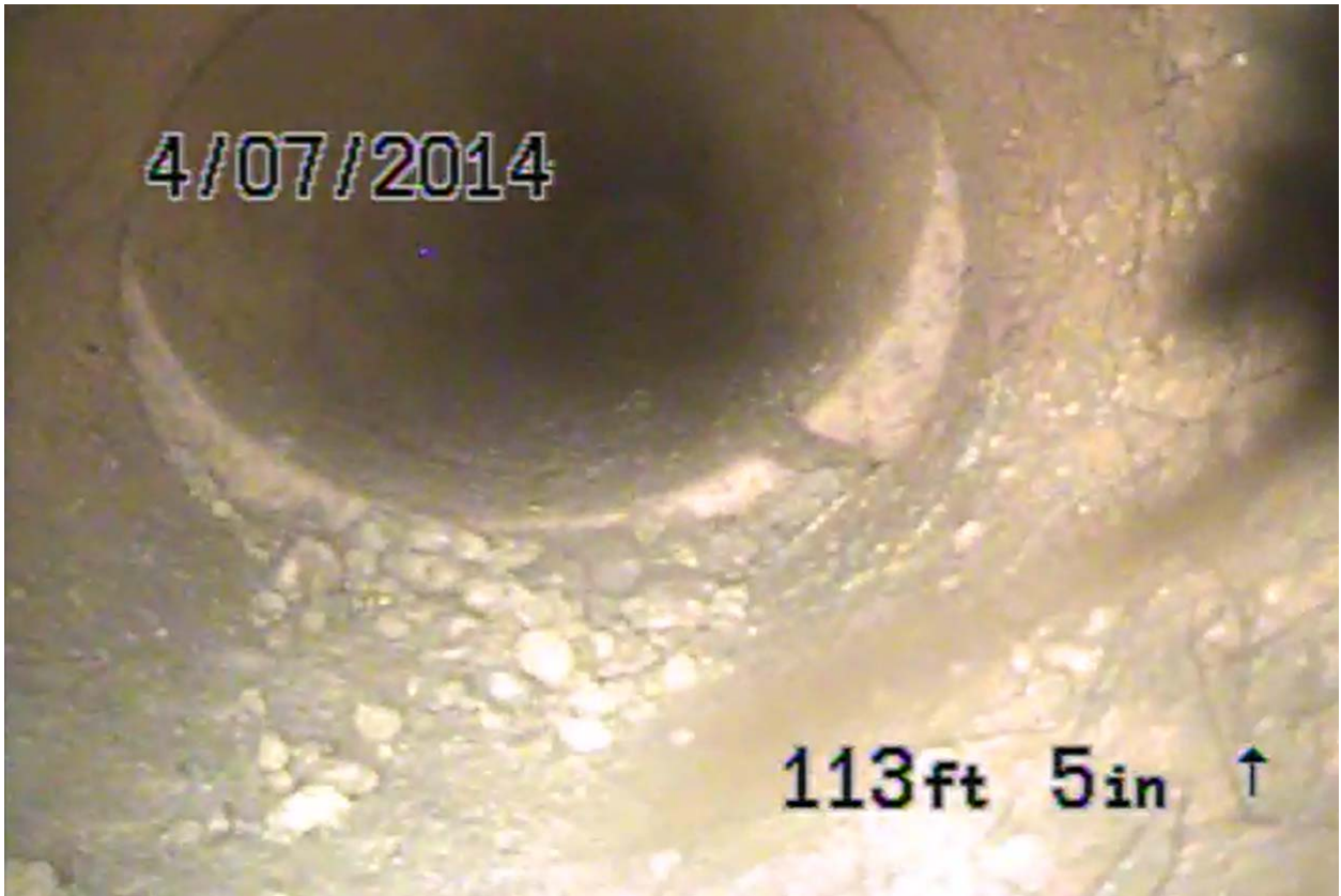
Screen shot 10: four-inch clay drain line 9 at Building 3 with off-set and cracked joint, approximately 113 feet from former sump
