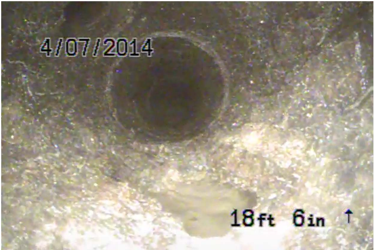
Screen shot 4: four-inch cast iron drain line 7 at Building 3 with unknown connection (left) and hole in bottom of pipe, approximately 18 feet from former sump
