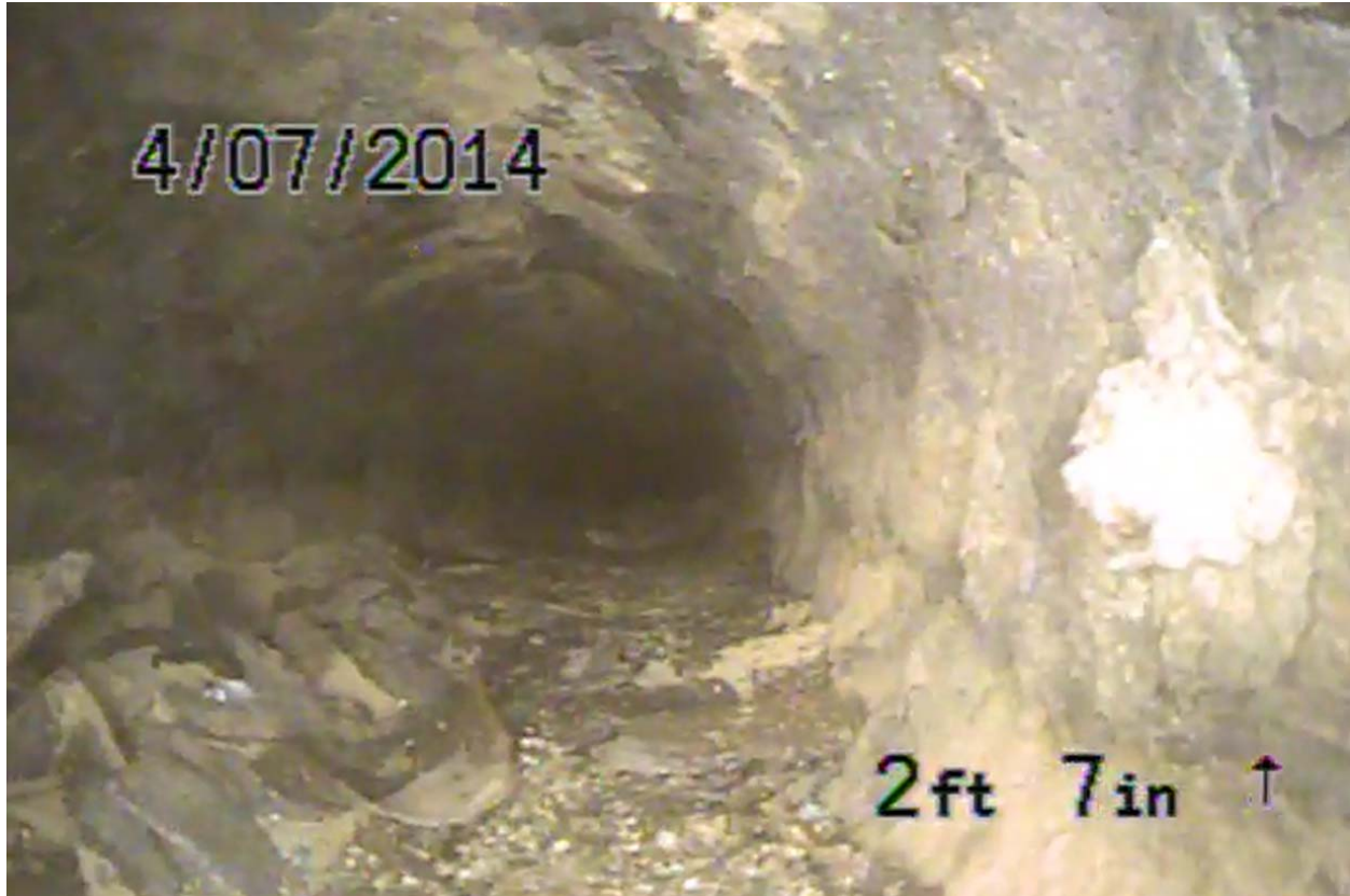
Screen shot 1: four-inch cast iron drain line 7 at Building 3 with wall deposits and sediment before cleaning
