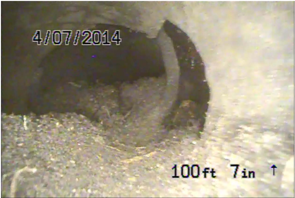
Screen shot 8: four-inch clay drain line 9 at Building 3 with potential break on right, approximately 100 feet from former sump
