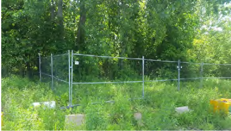
Photo 1 View looking south at the northeastern corner of the temporary fence installed at the Site.
