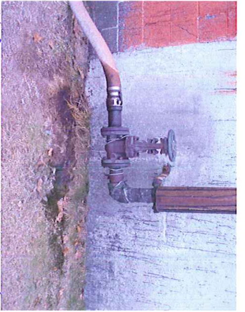
Fill for oil AST (Heating) Northside
