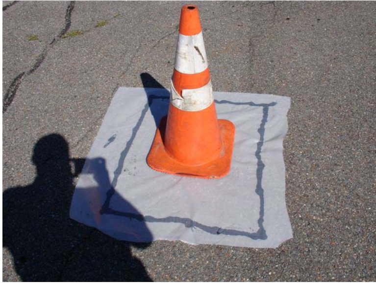
Area 1 Parking Lot Sinkhole
