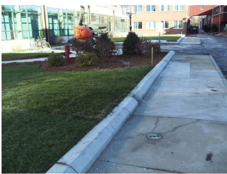
Steam Leak Area (RTN 3-31219)
